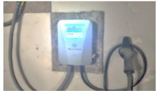
Utalika EV Charging point
